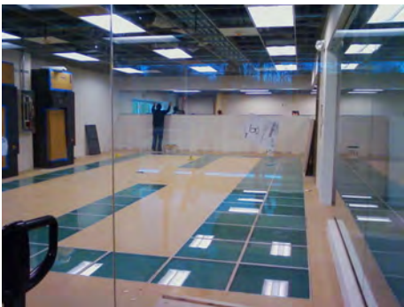
Before the racks are installed. Standard Tate Concore 1250 panel with SRF frames and laminated glass panels.
